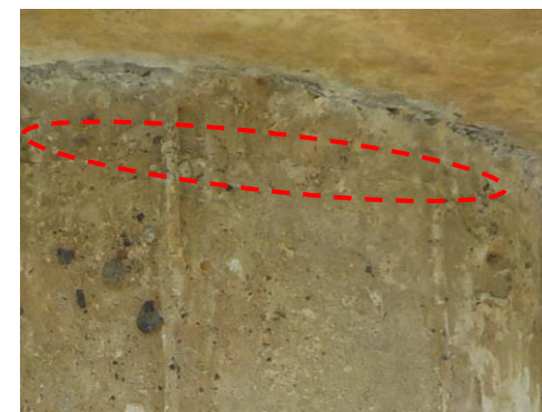
ひび割れ状況例 (No.2杭)
