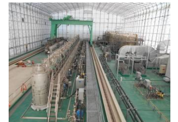
High-performance multi-nuclide removal equipment
