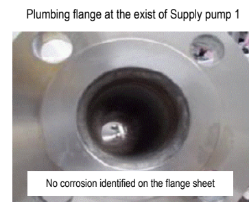
Plumbing flange at the exit of slurry transfer pump
