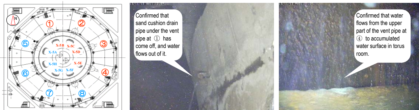
Figure 8: Water leakage from sand cushion drain pipe and upper part of vent pipe at Unit 1
