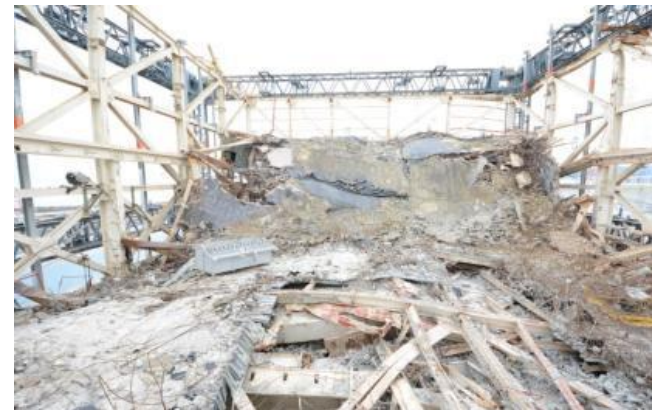
Actual collapsed roof on the south side
