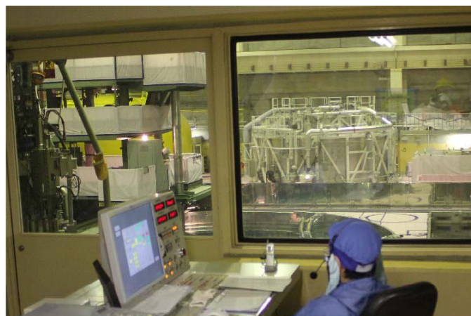
Monitoring operator to check entire status from the operation room of the fuel handling machine
