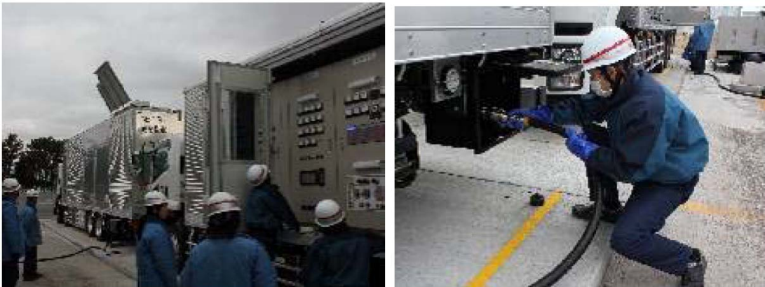
Scenes from a drill in Fukushima Daini NPS (Power Supply Drill using gas turbine generator vehicle)
