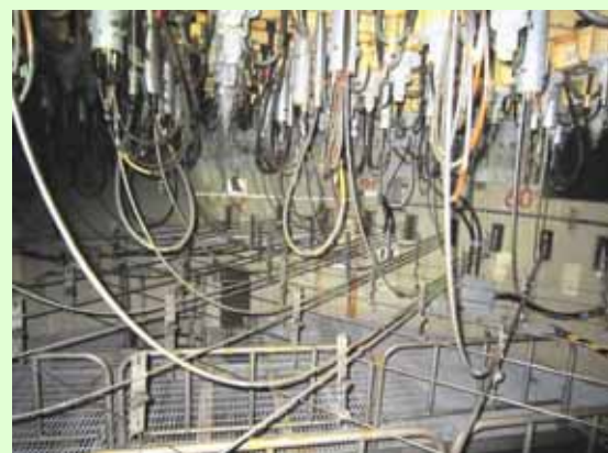
8. Pedestal (Base structure of RPV) (Photo taken on May 10, 2012)
