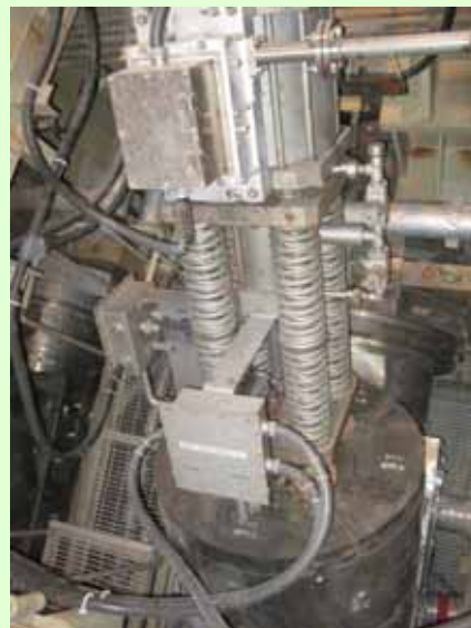
6. Main steam isolation valve (Photo taken on April 11, 2012)
