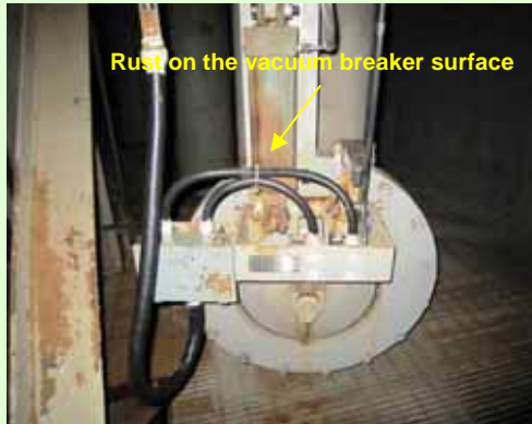
9. Rust on the vacuum breaker surface (Photo taken on April 17, 2012)
