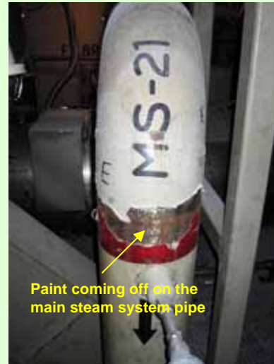
10. Paint coming off on the main steam system pipe (Photo taken on March 13, 2012)
