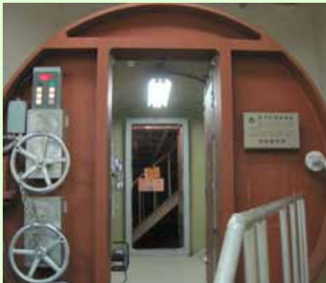
1. PCV entrance (Airlock for workers) (Photo taken on May 10, 2012)
