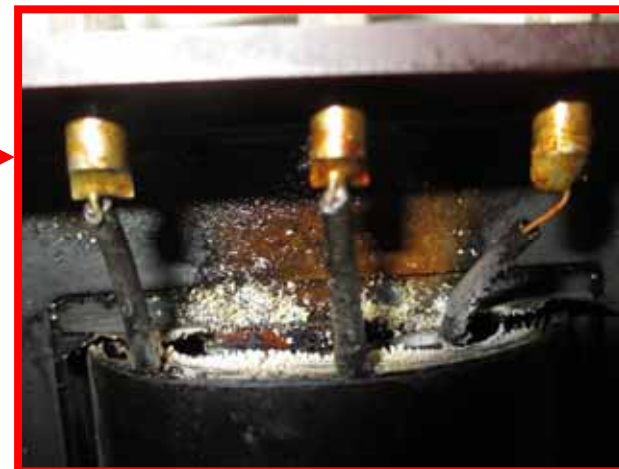
The inside of winding got heated up and insulating varnish is melted
