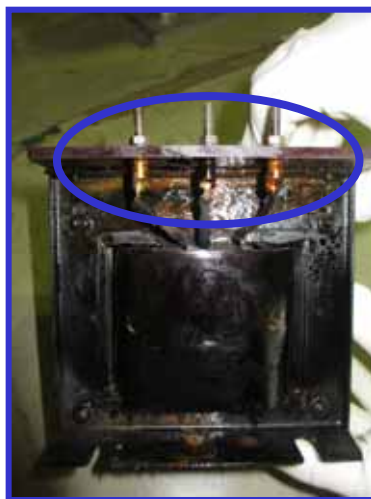
Terminal of the secondary winding (Photo taken from below the transformer)
