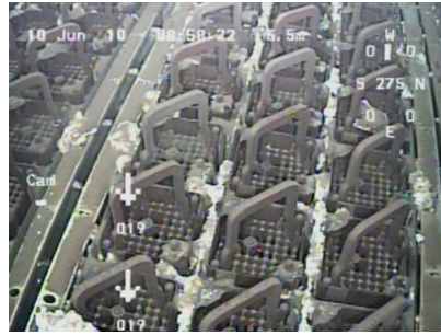
Fuel and top of fuel rack
