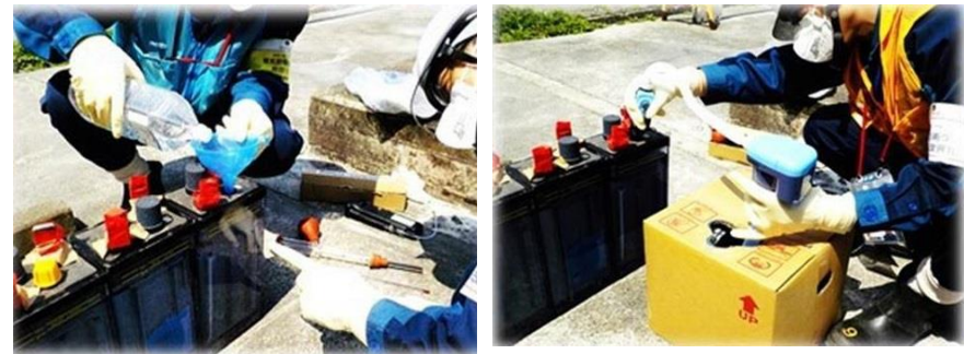
Replenishing liquid in storage batteries (Left: Prior to kaizen, Right: After kaizen)
