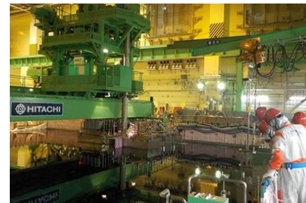
Fuel cleaning (Unit 7)
