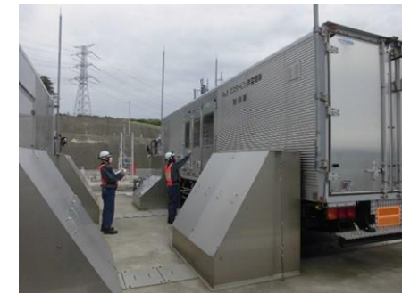
Gas turbine generator truck operation training
