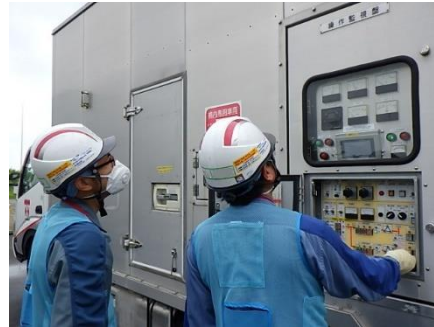
Voltage/frequency adjustment (power supply truck operation training)
