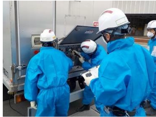
Power supply truck operation/connection training
