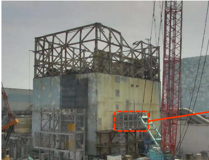
Photo 1. Unit 1 reactor building conditions (high-angle view)
