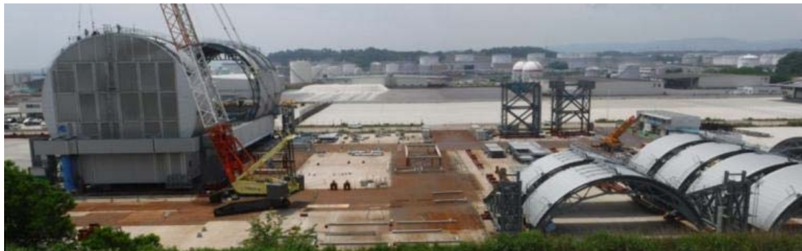
Training in the Onahama Port on the installation of a domed roof
